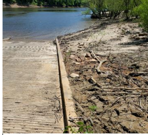
Seep entering river.
